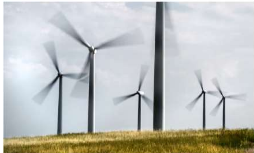
Combination of 221 Mitsubishi Heavy Industries 1-MW turbines and 53 GE 1.5-MW turbines at the Cedar Creek Wind Farm in Grover, Colorado. Photo by Dennis Schroeder, NREL 30593
